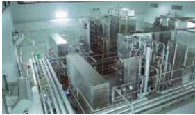
Fonterra's processing line protected by PCS100 AVC
